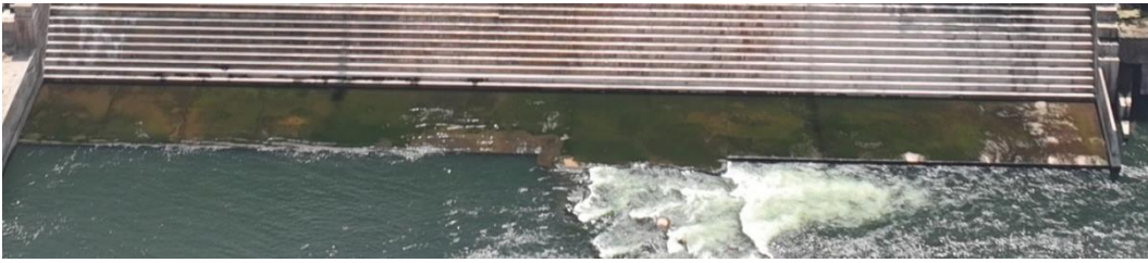
Figure 18. Bottom Slab status after seven years of duty operation
