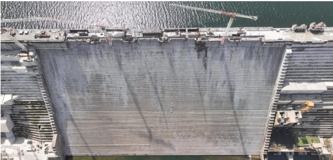
Figure 7 – GERD, Temporary stepped spillway, April 2024 general view after 7 years of heavy operation
